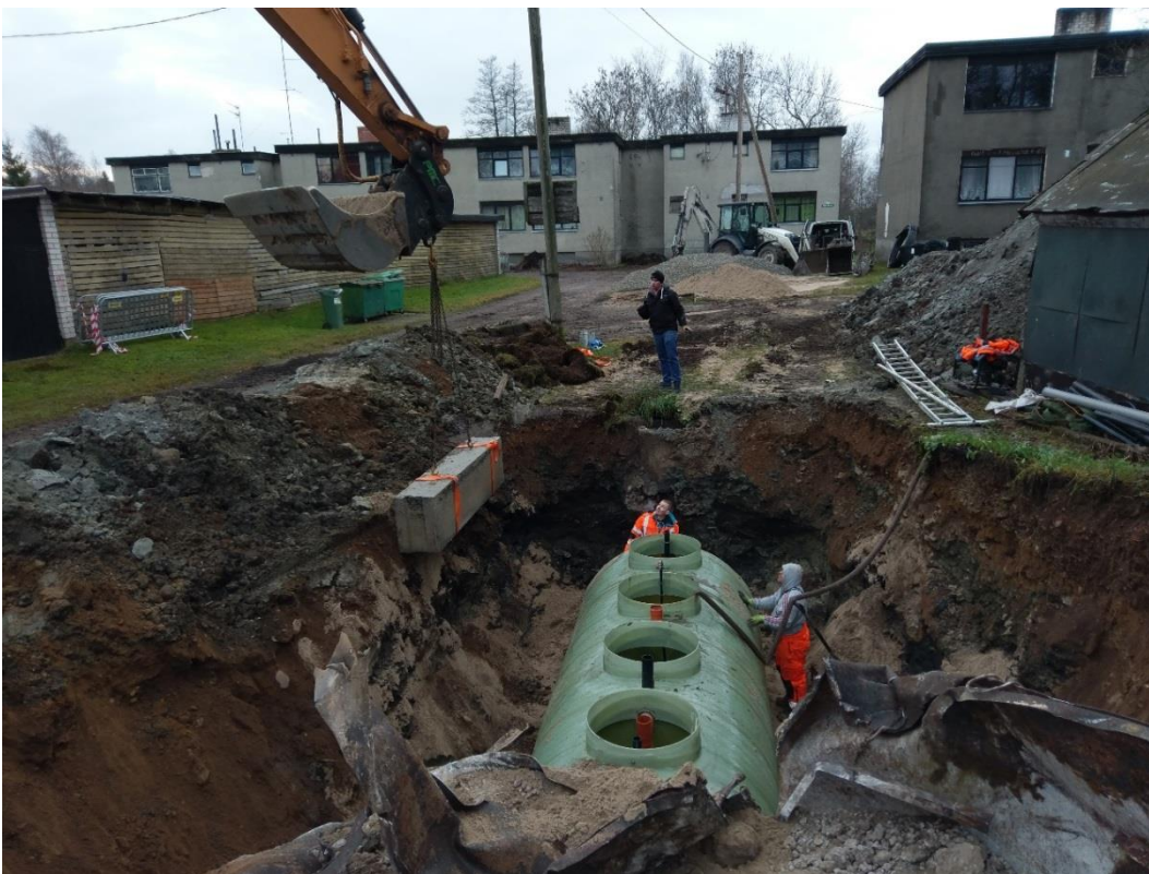
Picture 35. d. Materials, installations and devices used in the building process in Valkla village pilot.
