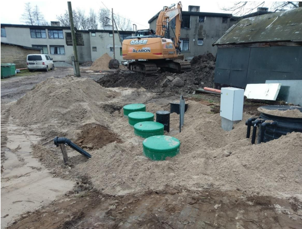
Picture 46. Valkla village pilot during the construction of WWTP and renovation of pipelines.
