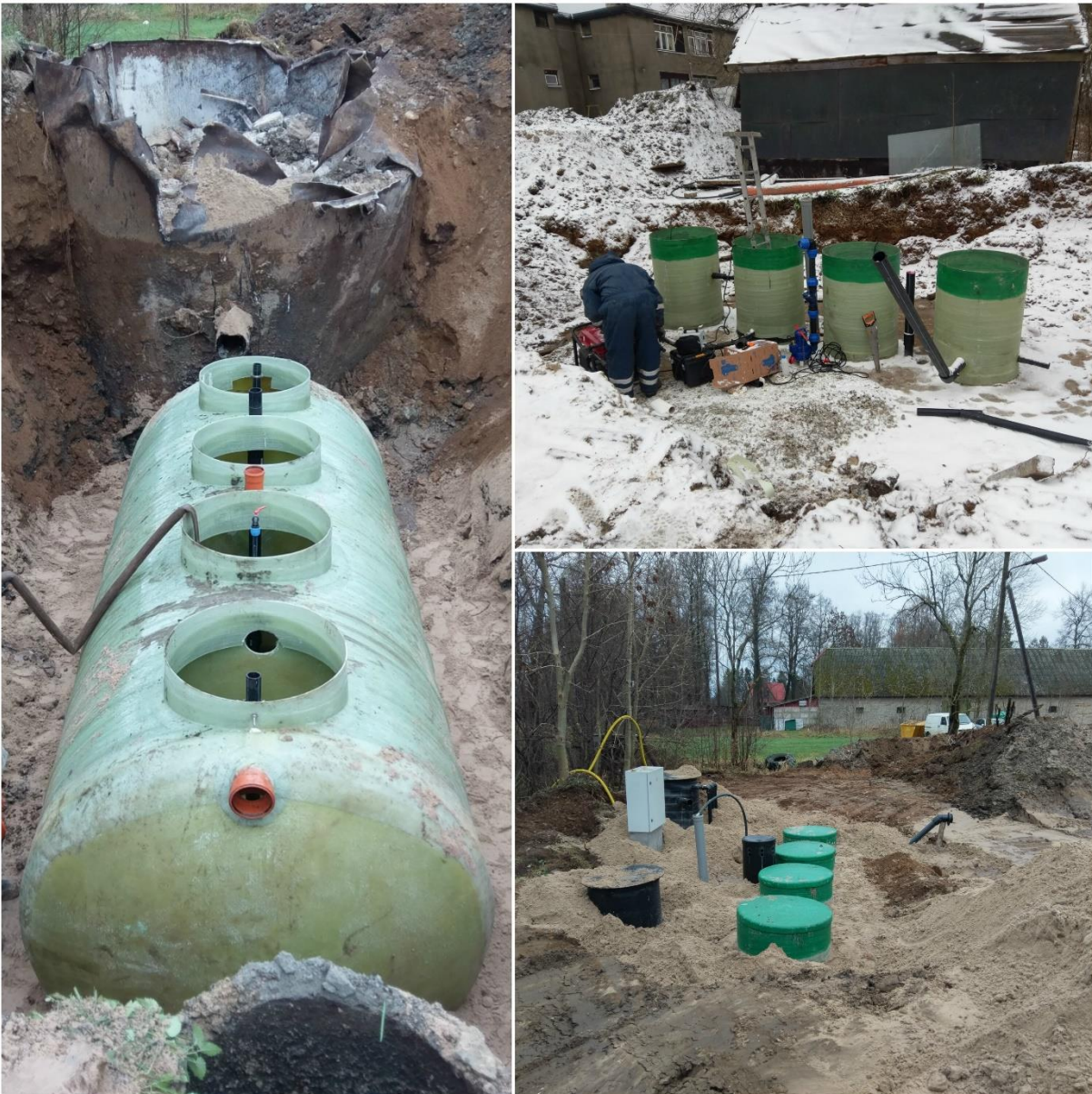
Picture 44. Valkla village pilot during the construction of WWTP and renovation of pipelines.
