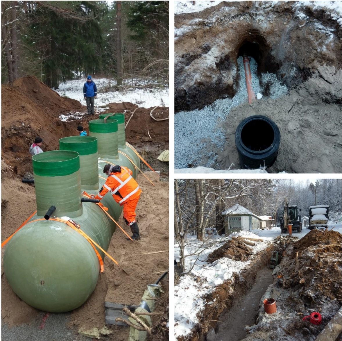
Picture 38. Kolgaküla village pilot during the construction of WWTP and renovation of pipelines.
