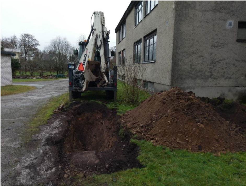
Picture 32. A. Materials, installations and devices used in the building process in Valkla village pilot.
