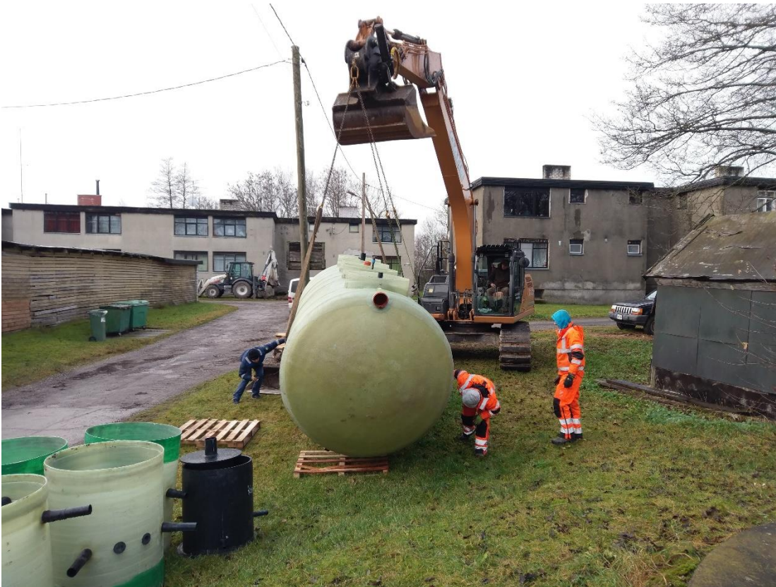
Picture 33. B. Materials, installations and devices used in the building process in Valkla village pilot.
