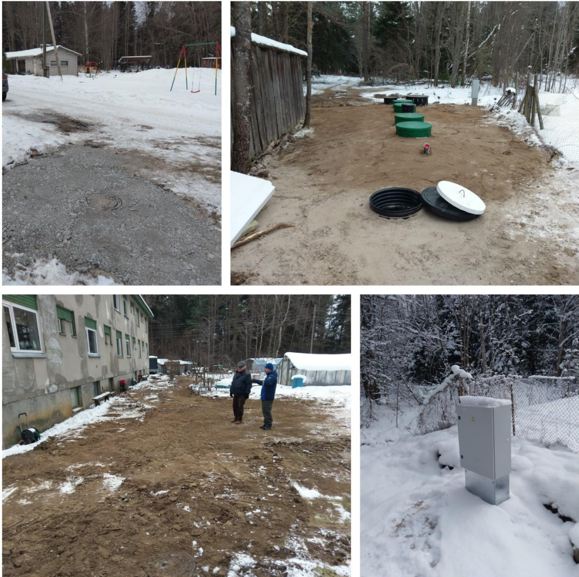
Picture 40. Kolgaküla village pilot after construction of WWTP and renovation of pipelines.
