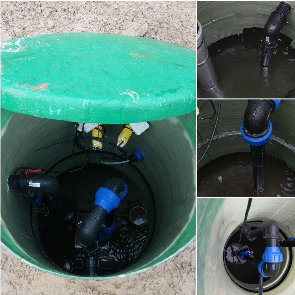
Picture 45. Valkla village pilot after the construction of WWTP and renovation of pipelines.
