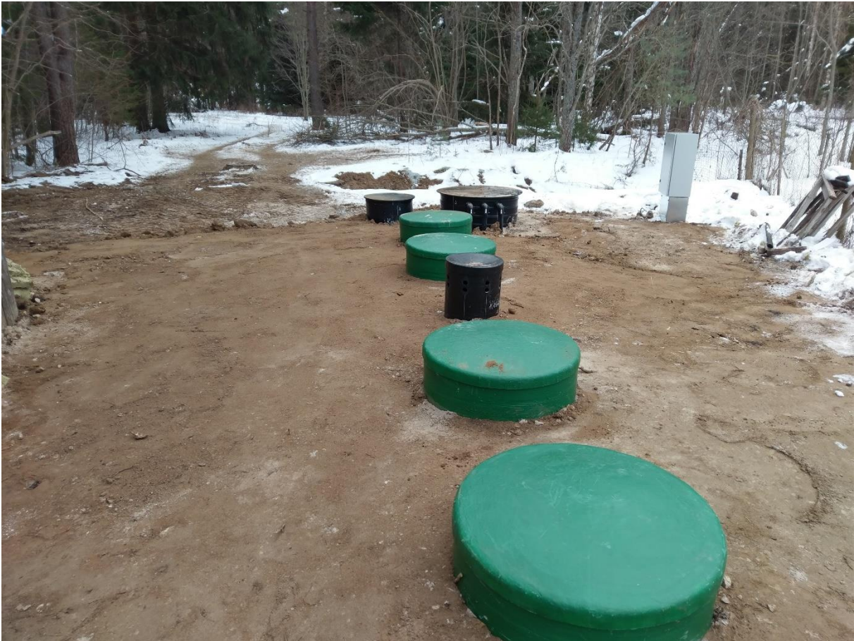
Picture 41. Kolgaküla village pilot after construction of WWTP and renovation of pipelines.
