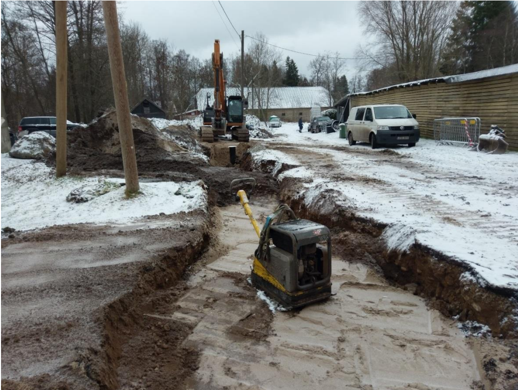
Picture 47. Valkla village pilot during the construction of WWTP and renovation of pipelines.
