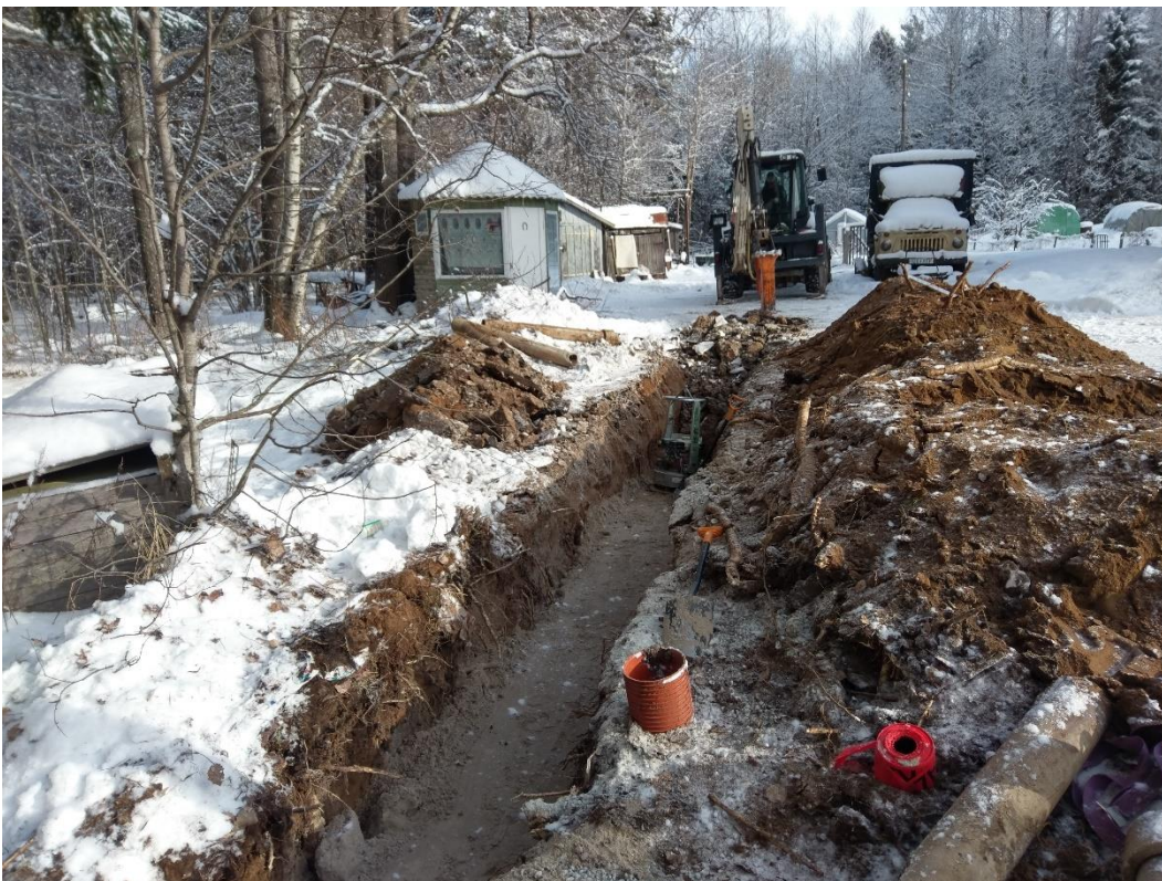
Picture 31. Materials, installations and devices used in the building process in Kolgaküla village pilot.
