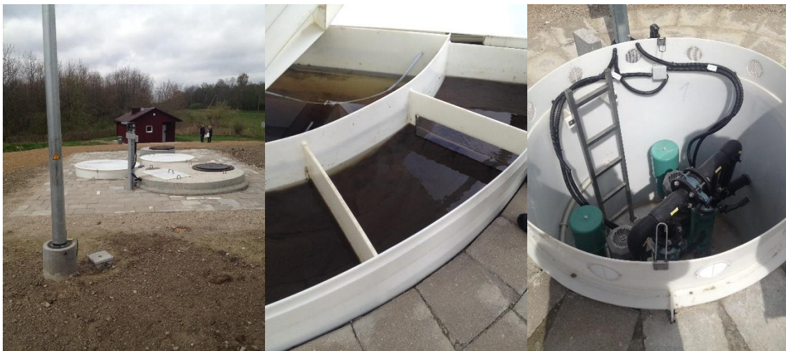
Picture 20. The new installed system.
