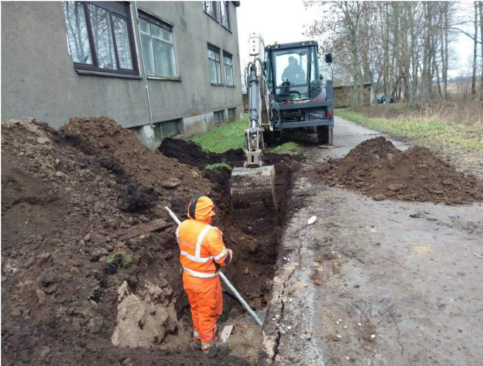
Picture 34. c. Materials, installations and devices used in the building process in Valkla village pilot.
