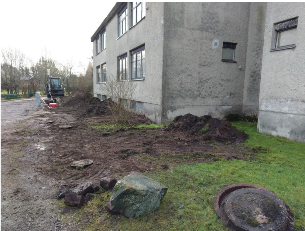
Picture 49. Valkla village pilot during the construction of WWTP and renovation of pipelines.
