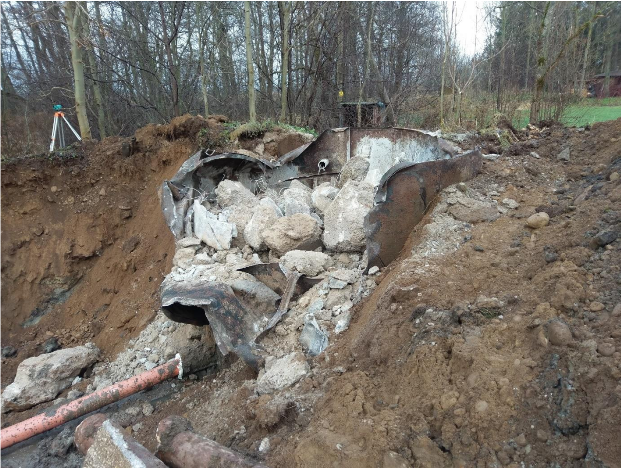
Picture 43. Valkla village pilot before construction of WWTP and renovation of pipelines.
