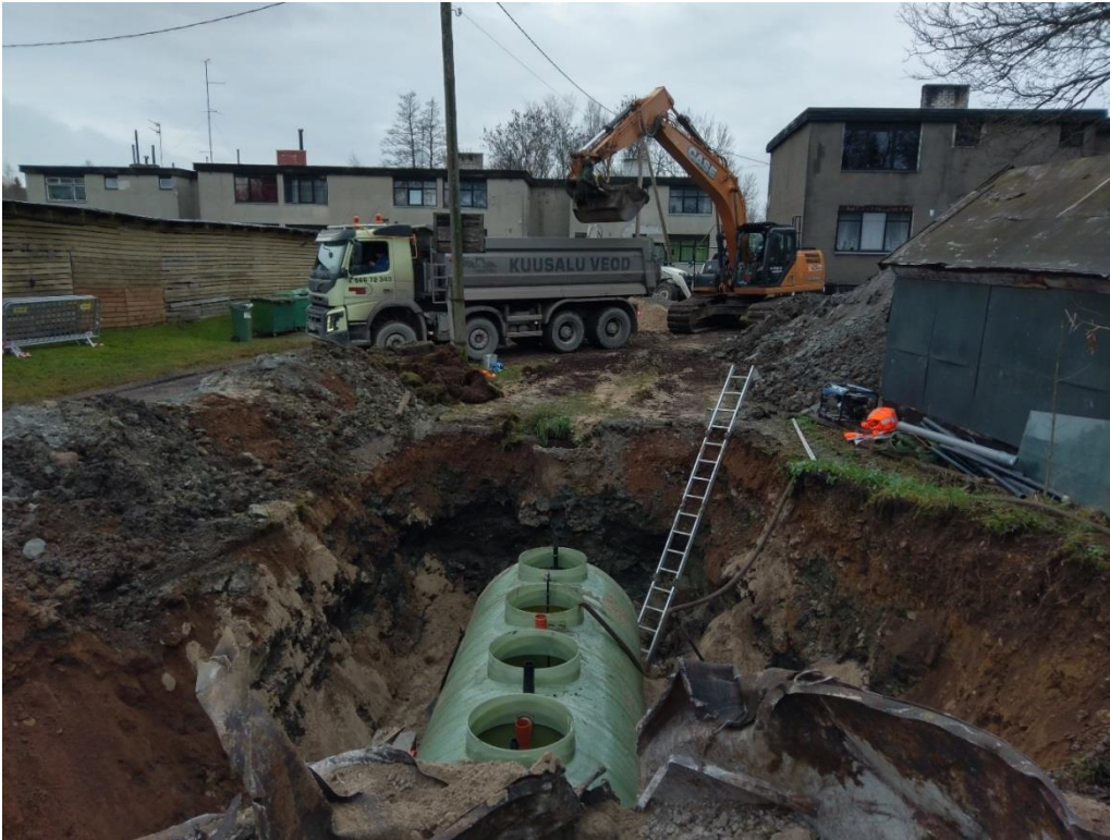
Picture 48. Valkla village pilot during the construction of WWTP and renovation of pipelines.
