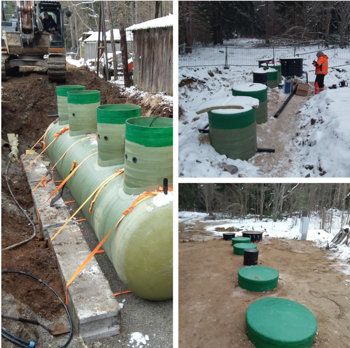
Picture 39. Kolgaküla village pilot during and after construction of WWTP and renovation of pipelines.
